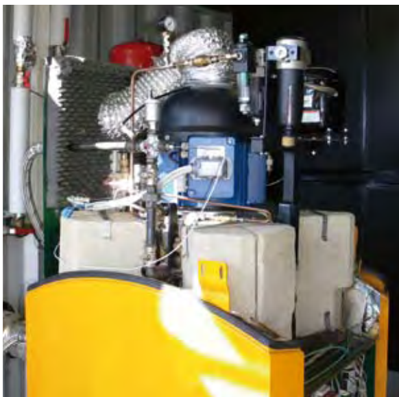
Fig. 2: Conception and control of a miniature micro-CHP system using wood pellets as the fuel. The goal was to maximise the electricity yield with a sophisticated energy management concept and flexible use of waste heat with highly efficient heat storage and supply. The photo shows the Stirling engine and the pellet burner in the laboratory. (Photo: Stirling Power Module GmbH).
