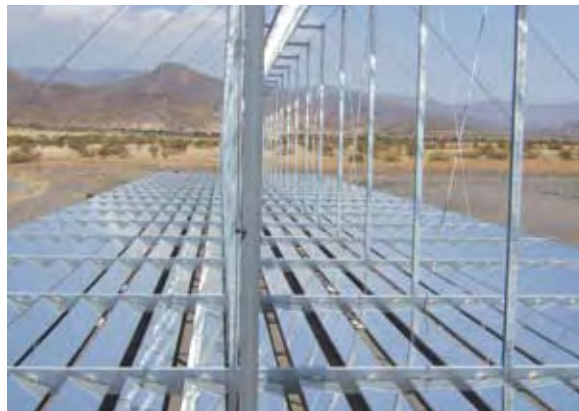
Fig. 3: FRESDEMO test collector at the Plataforma Solar de Almería, Spain. Measurement of this collector serves as the basis for techno-economic evaluation of Fresnel technology (base case).
